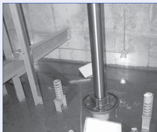
Elevator shafts at both CAPITAL CARE Grandview and CAPITAL CARE Lynnwood were flooded.
