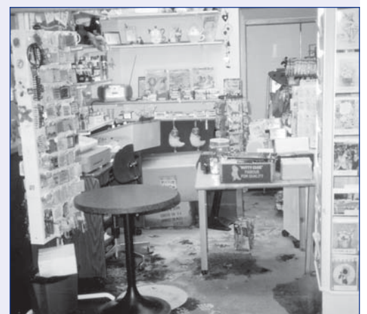
After the flood waters receded, a layer of dirt and leaves covered the first floor at CAPITAL CARE Grandview .
